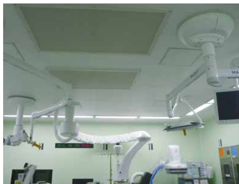
Fig 1. Highly hygiene operating room without any obstructions under the high efficiency particulate air
